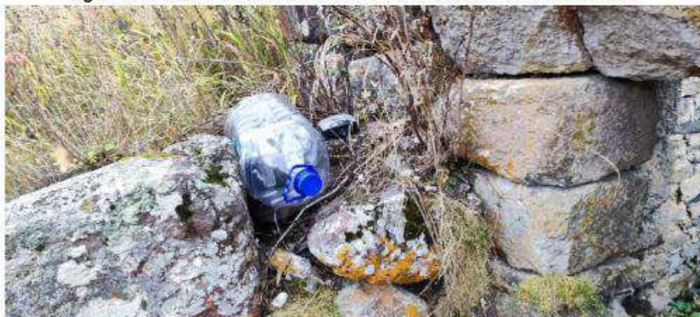
Figure 6.1: Vibration monitor SWARM was installed outside on the wall of the Tower
