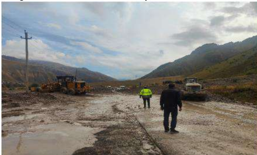
Figure 35: CRTG and PMCSC helped to remove land silide from E-117
